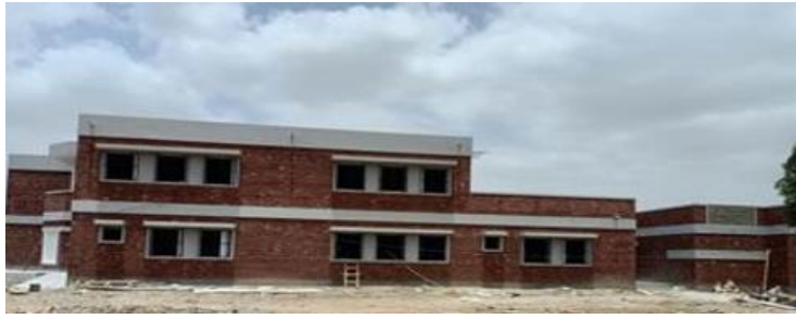
Picture 12: The construction of a secondary school in partnership with The Citizens Foundation
