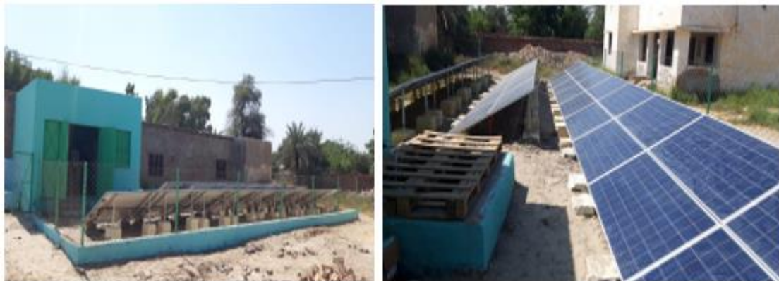
Picture 8: Solar powered RO Plant installed in district Sanghar
